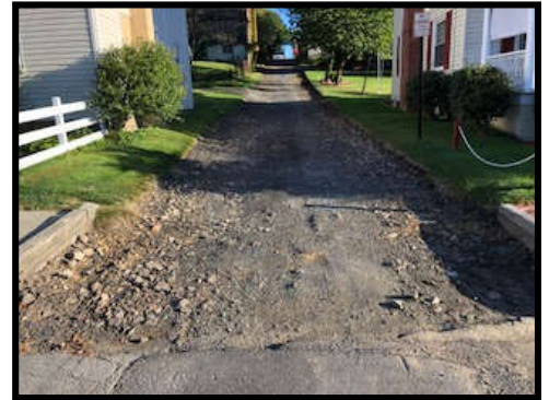
Block of Poplar Street remains completely destroyed lacking even a base.
