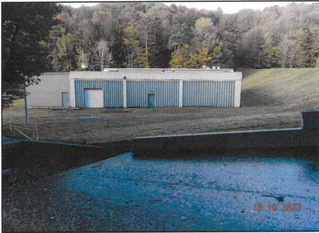
Photo 17: Recently Removed Upper Section of the Western Spillway Wall (EMA operational staff removed portion of wall in 2019)
