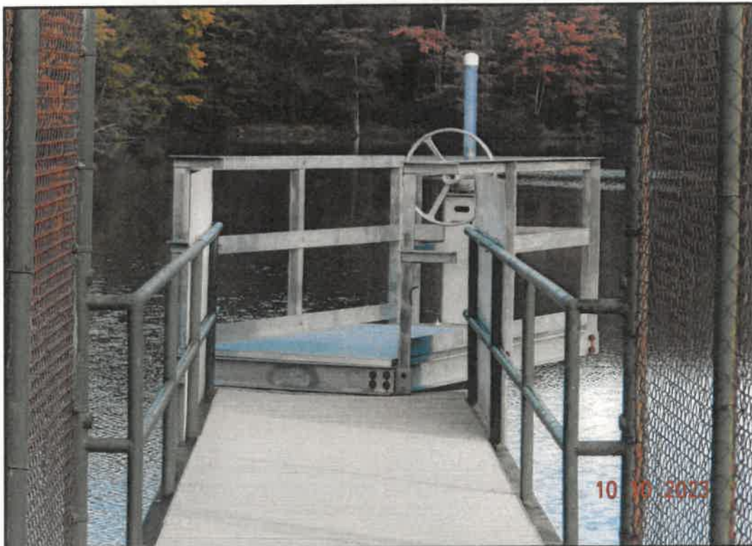
Photo 16: Newly installed primary closure drain valve operator and access platform. (20" Stainless Steel Sluice Gate)
