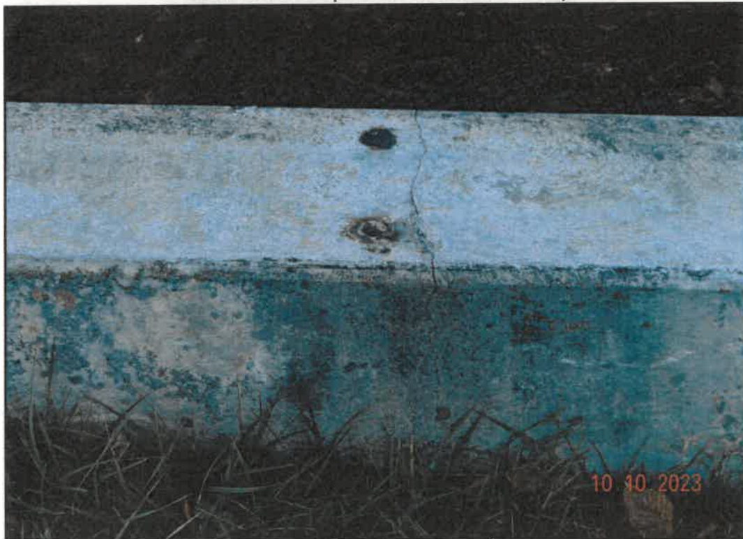
Photo 18: Hairline Cracking in Western Spillway Wall
