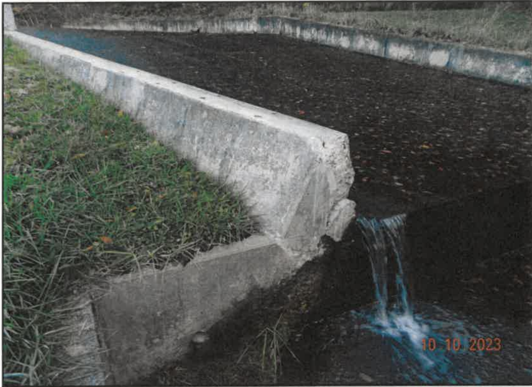
Photo 13: Recently Removed Upper Section of the Western Spillway Wall (EMA operational staff removed portion of wall in 2019)
