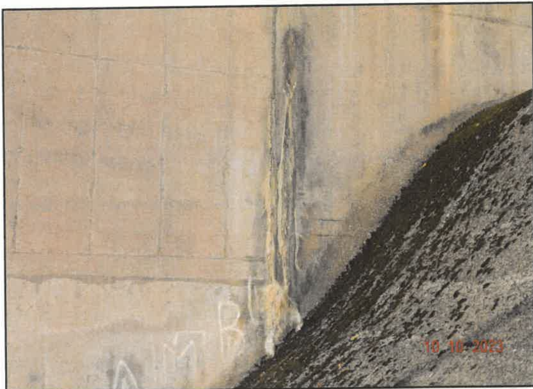
Photo 22: View of Seepage through Western Spillway Wall approx. 10' below Weir. Note that most of the Discharge is not in the Wall Joint. (note. no liquid seepage was observed, only
