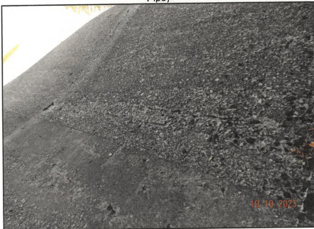
Photo 34: Exposed Reinforcement Bar in Face of Ogee
