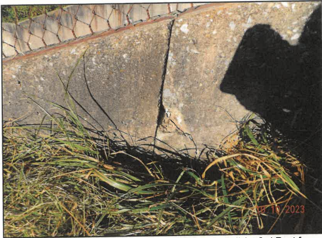
Photo 35: Spalling and Cracking Concrete on Eastern Wall (at 3rd Post from Crest)
