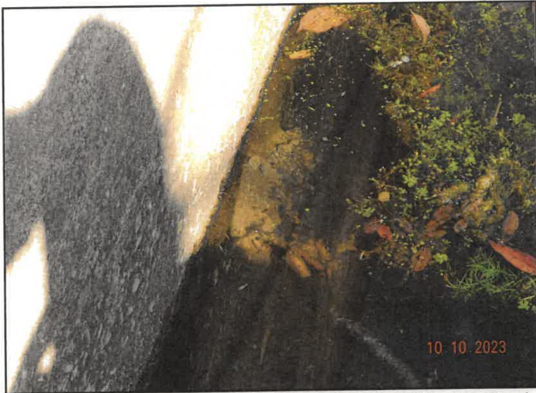
Photo 33: Backfill at Base of Weepole on Western Abutment Wall (Possible Collapsed Pipe)
