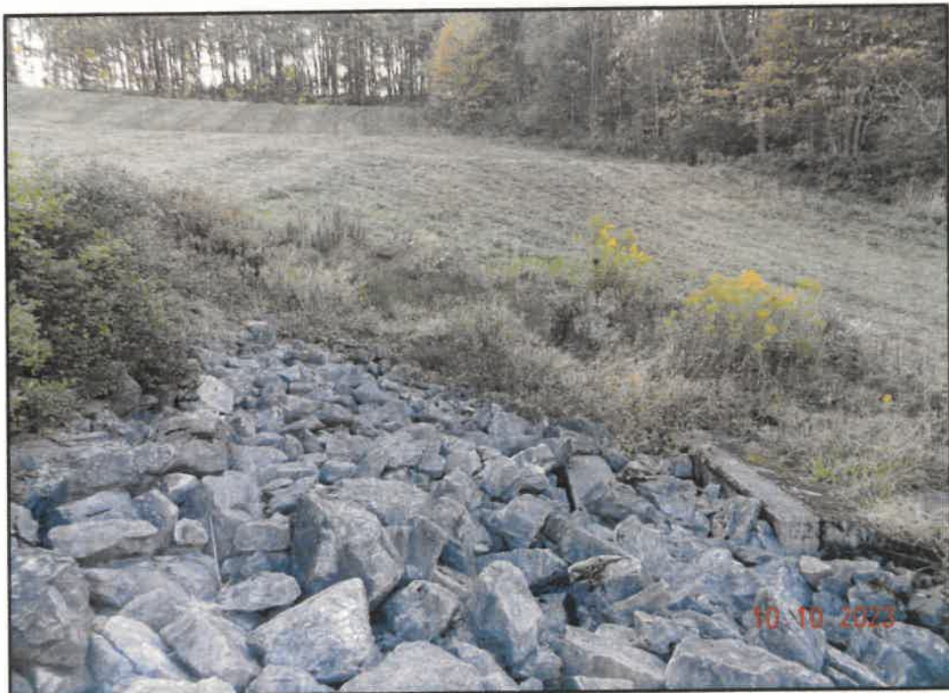
Photo 18: View of "Wet Area" Adjacent to Junction Box (dry this year)
