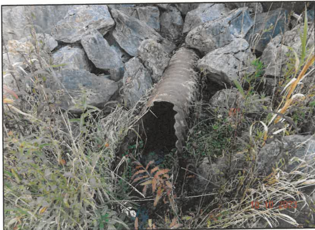
Photo 26: Corroded 15" CMP passing through stilling basin weir wall.
