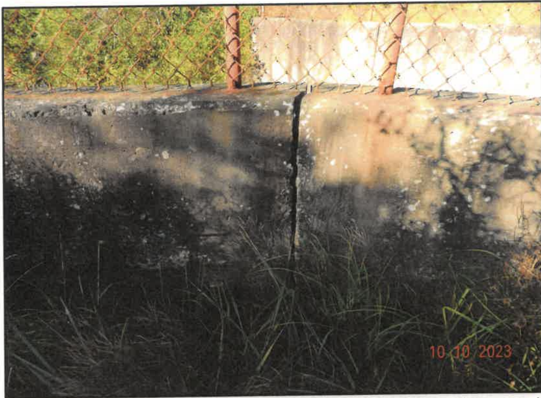
Photo 29: Joint with Active Flow of Water in Eastern Abutment Wall adjacent to Wet Area (Back Face View)
