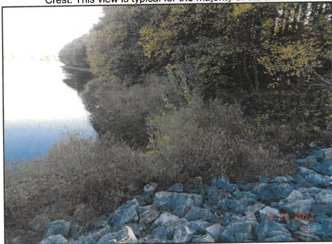
Photo 24: View of Overgrown Brush along Southeastern Upstream Embankment.
