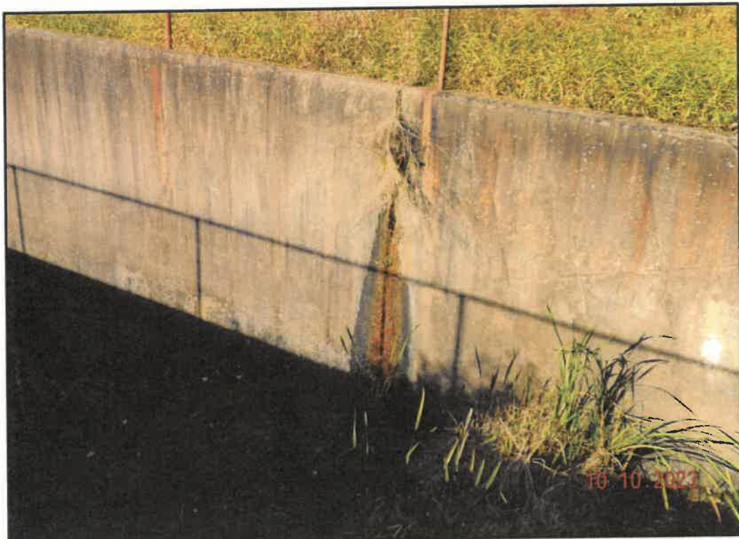
Photo 20: View of Seepage area on Western Wall Above Stilling Basin
