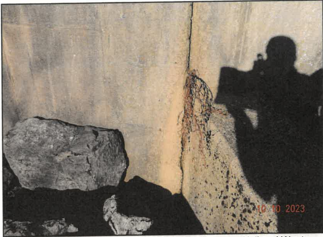
Photo 21: View of Seepage area between Stilling Basin Weir Wall and Western Abutment
