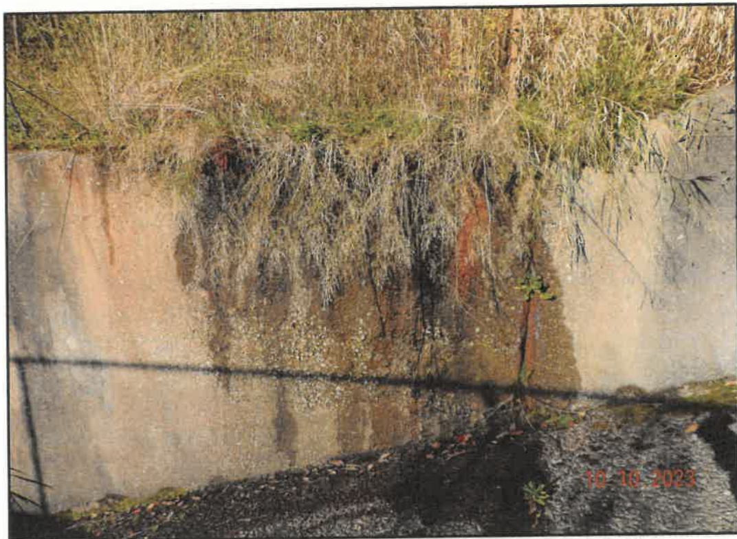
Photo 32: View of Seepage Area on Western Wall Above Stilling Basin
