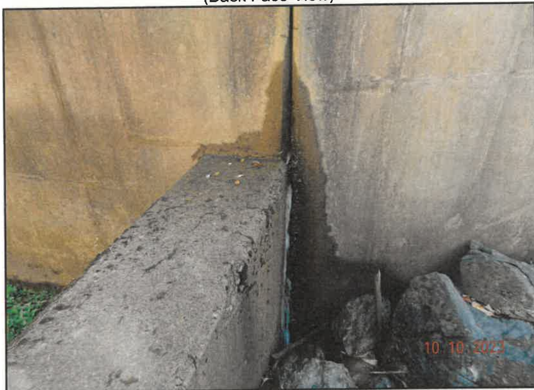
Photo 30: Joint with Active Flow of Water in Eastern Abutment Wall adjacent to Wet Area (Front Face View)
