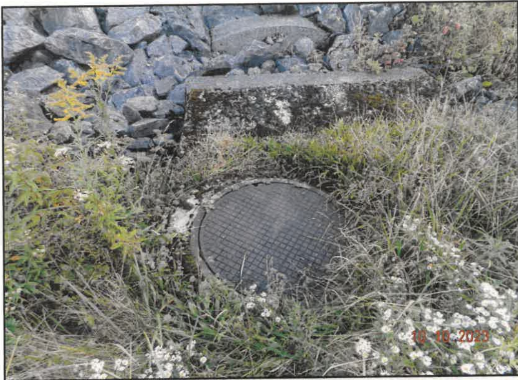
Photo 17: View of Junction Box for Drain Pipe Extension at Toe of Embankment
