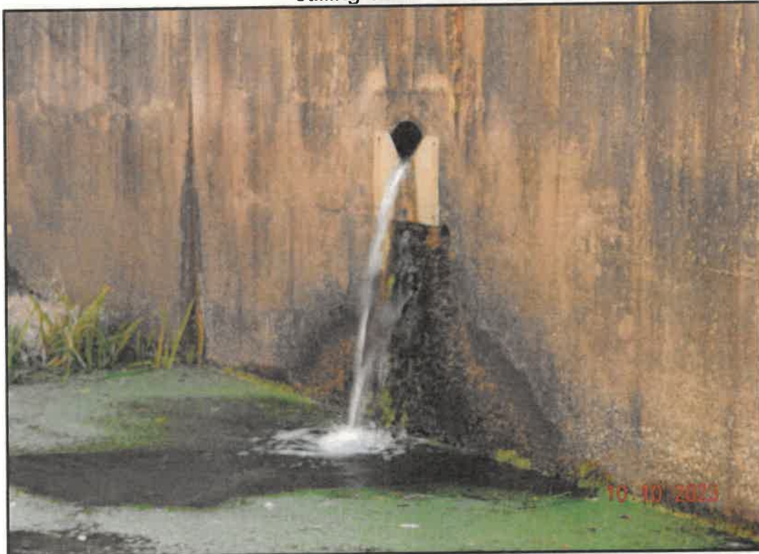
Photo 16: View of Weired Seepage Outlet through Eastern Spillway Wall. (Note, water seeping behind and under weir plate)
